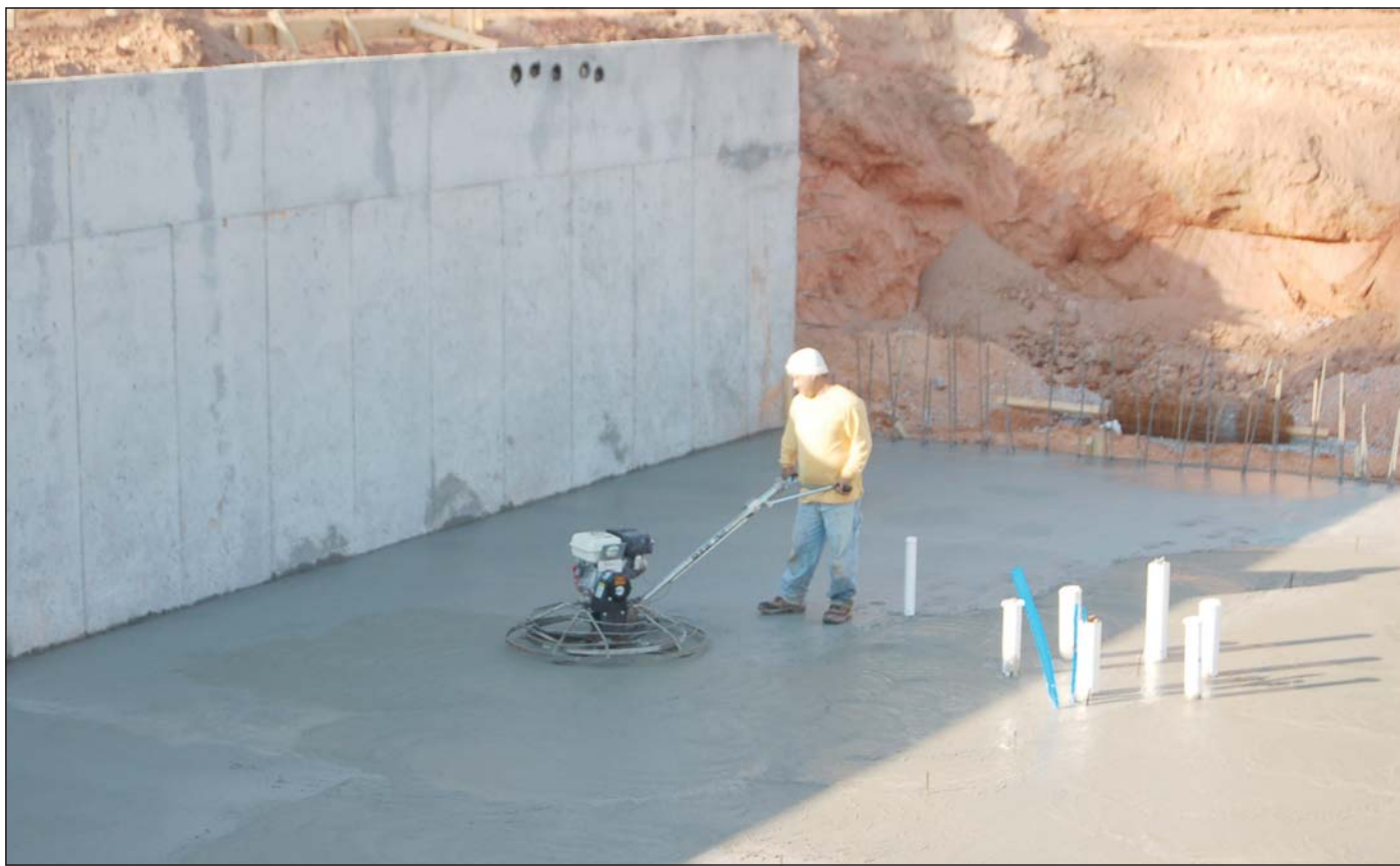
A workman smooths fresh concrete at the base of one of the five buildings in the first phase of the 54-unit Candler Point mixed-use development on South Rainbow Drive in Decatur.
